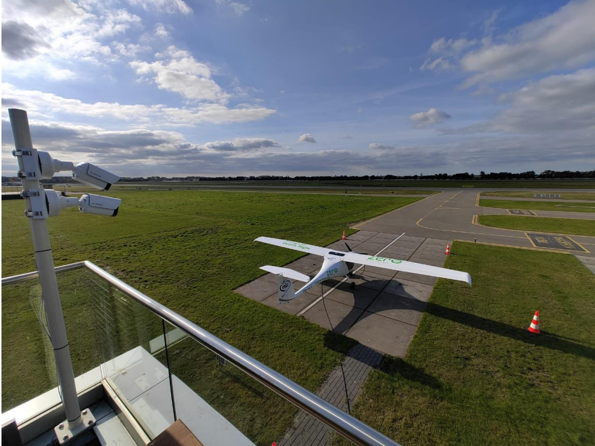
Figure 3. Bosch A.I. smoke and fire detection cameras installed at RAC for TULIPS demo (img src Jens van den Berg)
